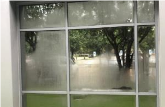
Exterior condensation before WinSert Plus installation.
