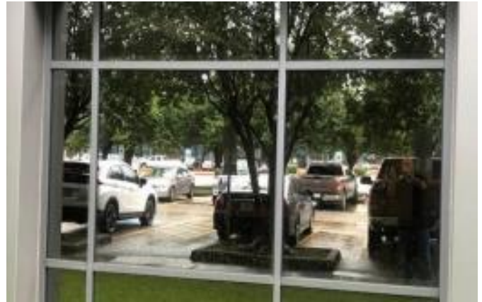
Condensation eliminated after WinSert Plus installation.
